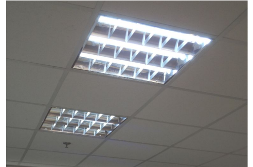
Typical case of one-to-one replacement
